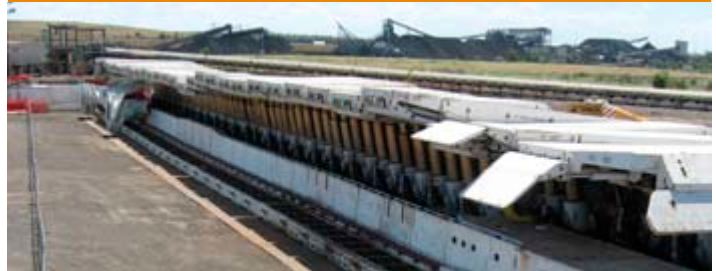
Joy electronic roof supports at Moranbah North Mine.
