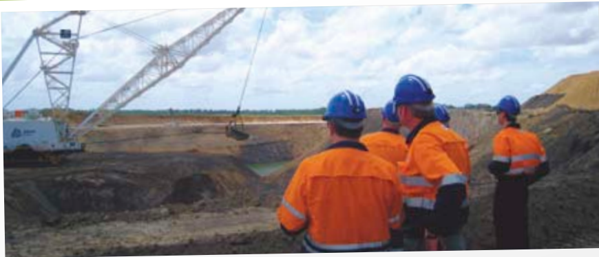
Alisdair Gibbons, Seamus French, Ian Cockerill and Ian Botha overlook the new Bucyrus dragline undergoing commissioning trials.
